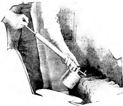
FIG. 23.—With a sprayer, whether hand, foot, or motor-driven, it is easy to finish radiators.
