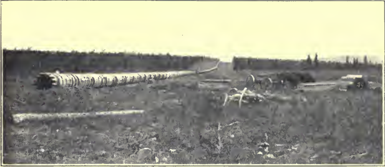
WOODEN STAVE PIPE-LINE.
