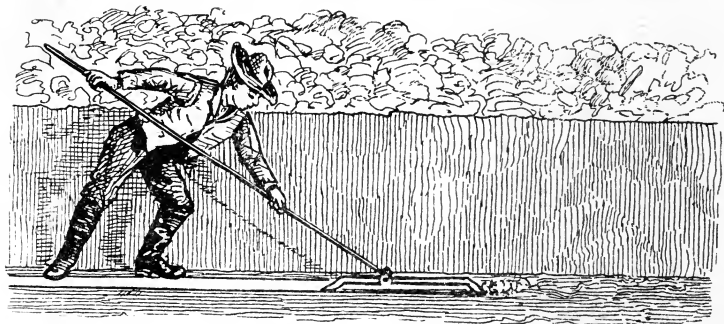
Fig. 26.—Position of workman using the “bottoming-scoop” or “groove-cutter.” Here he stands in the ditch, one side removed.
