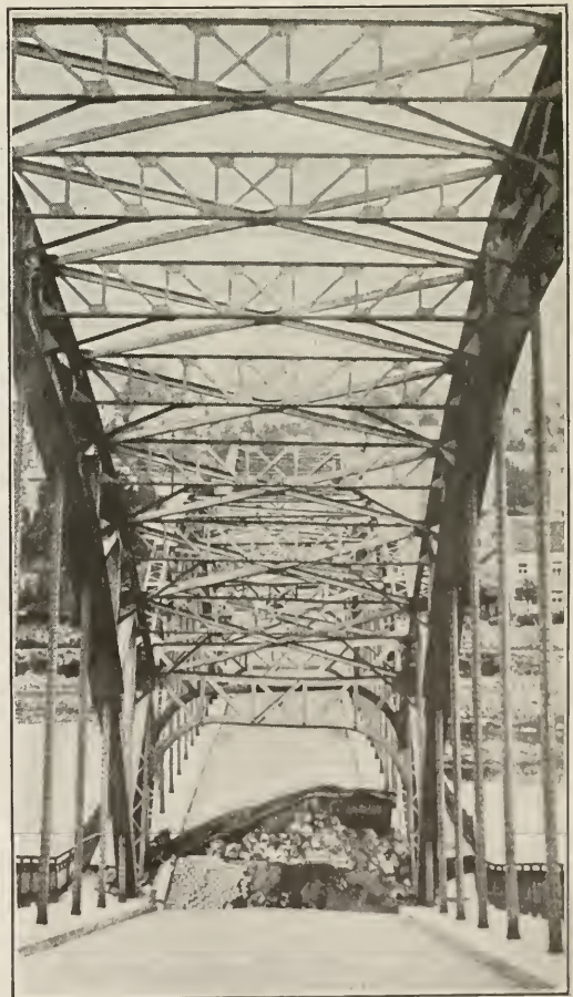
BRIDGE OVER THE MEUSE, Showing the destroyed centre.
