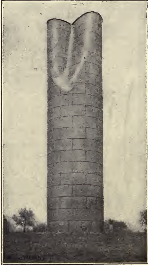
FIG. 7.—VIEW SHOWING EFFECT OF WIND ON STAND-PIPE AT LINCOLN, NEB. ( Engineering News. )
