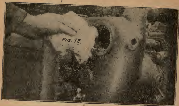
Fig. 72. 3d. Put waste in the hole to catch any valve grinding compound or sediment that may drop.
