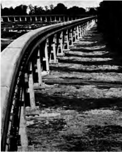
Close-up of part of the beam track of the Alweg experimental line at Cologne-Fühlingen. (Photo: Alweg)
