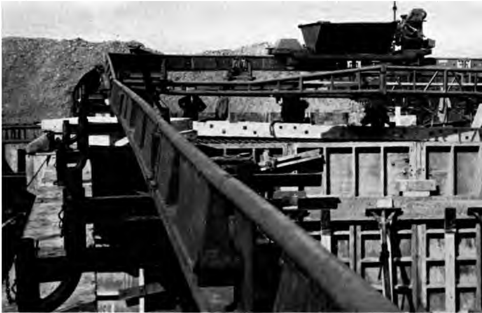
A standard gearbox drive Mono-Rail industrial car crossing a Mono-Rail bridge. The track supports can be seen clearly in the foreground. (Photo: Road Machines (Sales) Limited)
