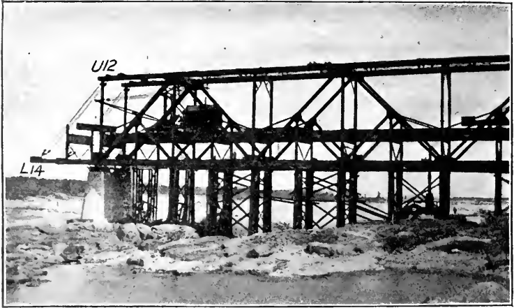
Fig. 3:—Southern anchor-span erected; and beginning of cantilever-erection, shewing temporary supports for panel-points L14 .
