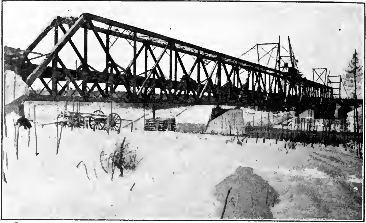
Fig. 11:—View of bridge from south shore before cableway and traveller had been dismantled. Note that the lower members of the portal-struts and sway-bracing are missing; they were omitted temporarily for the accommodation of the derrick-car.
