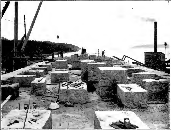
South Main Pier in Course of Construction. Note the Alternate Headers and Stretchers in Granite Face and Vertical Bond Stones projecting through the Courses.
