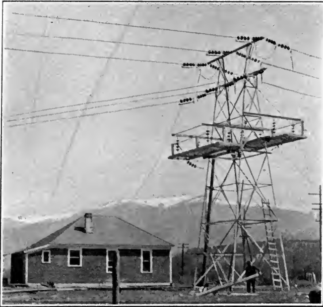
FIG. 103.—Dead-end switch tower with insulated platform.
