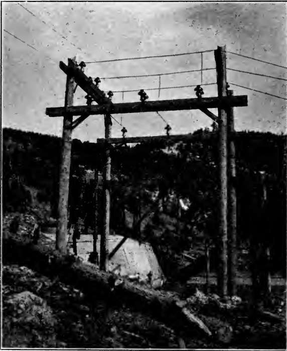
FIG. 111.—Wood pole junction or dead-end structure.
