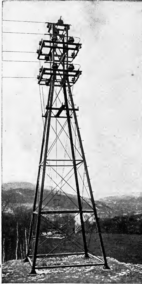
FIG. 119.—Special heavy-angle tower—Hoosac Tunnel electrification.
