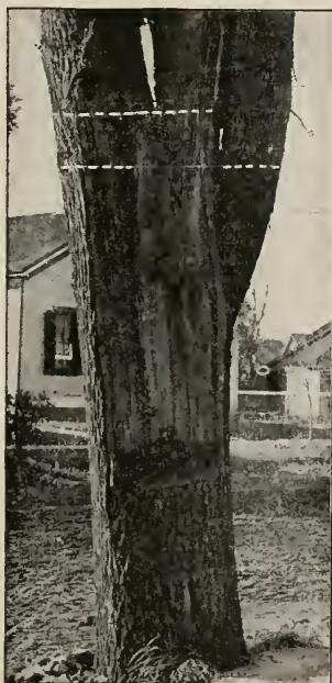
Photo 39 A Bolt is Needed.
