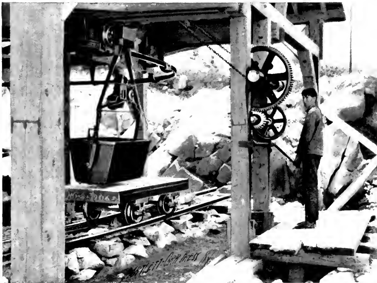
Mechanism for transferring Buckets to and from Surface Cars at Loading Terminal of line built for The Farnam-Cheshire Lime Co., Cheshire, Mass.
