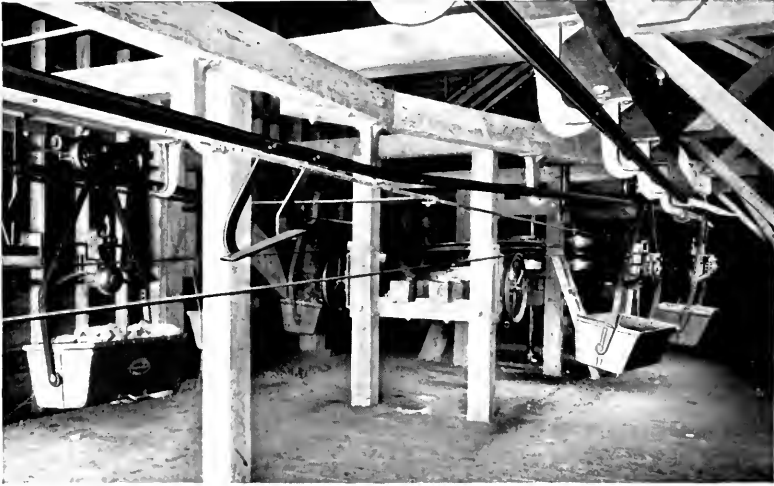
Loading Terminal, Trenton-Bleichert Tramway of the United States Mining Company, Bingham, Utah. Showing Detacher and Loaded Carrier in position for attaching to the Traction Rope.
