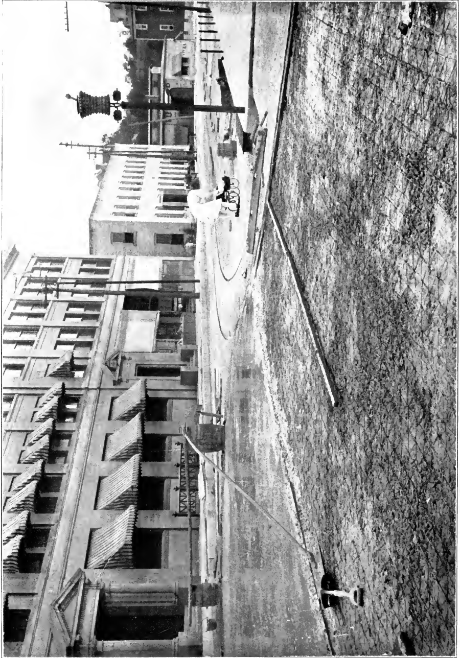
Reinforced Concrete Pavement, Plymouth, Wis. 100,000 Square Feet Triangle Mesh Reinforcement Used. Designing Engineer: W. G. Kirchoffer, Madison, Wis.
