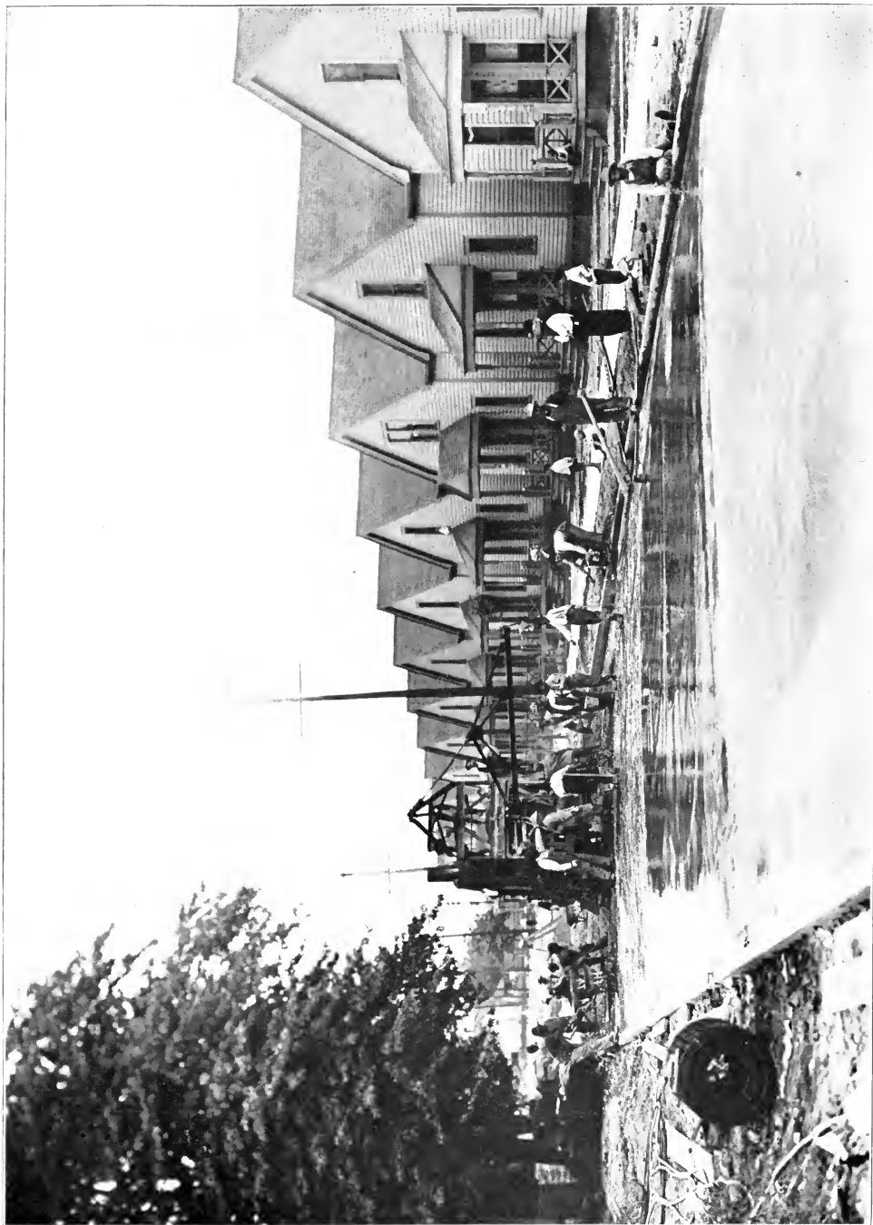
Reinforced Concrete Pavement, Hamtramck, Mich. 106,000 Square Feet Triangle Mesh Reinforcement, Style No. 28 Used. Contractor: R. D. Baker Co., Detroit, Mich.
