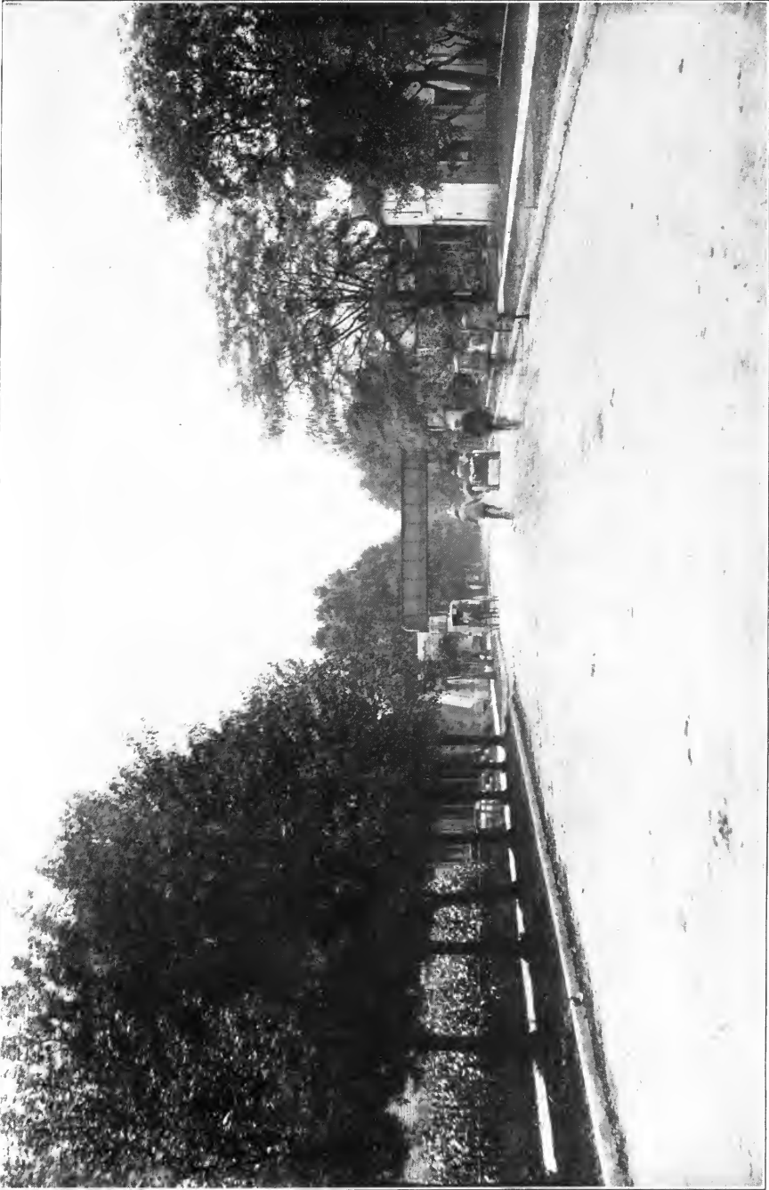
Reinforced Concrete Pavement, Connerville, Ind. 585,000 Square Feet Triangle Mesh Reinforcement Used. City Engineer: W. F. Ridpath. Contractors: Greenwood, Connor, Boots & Gant.
