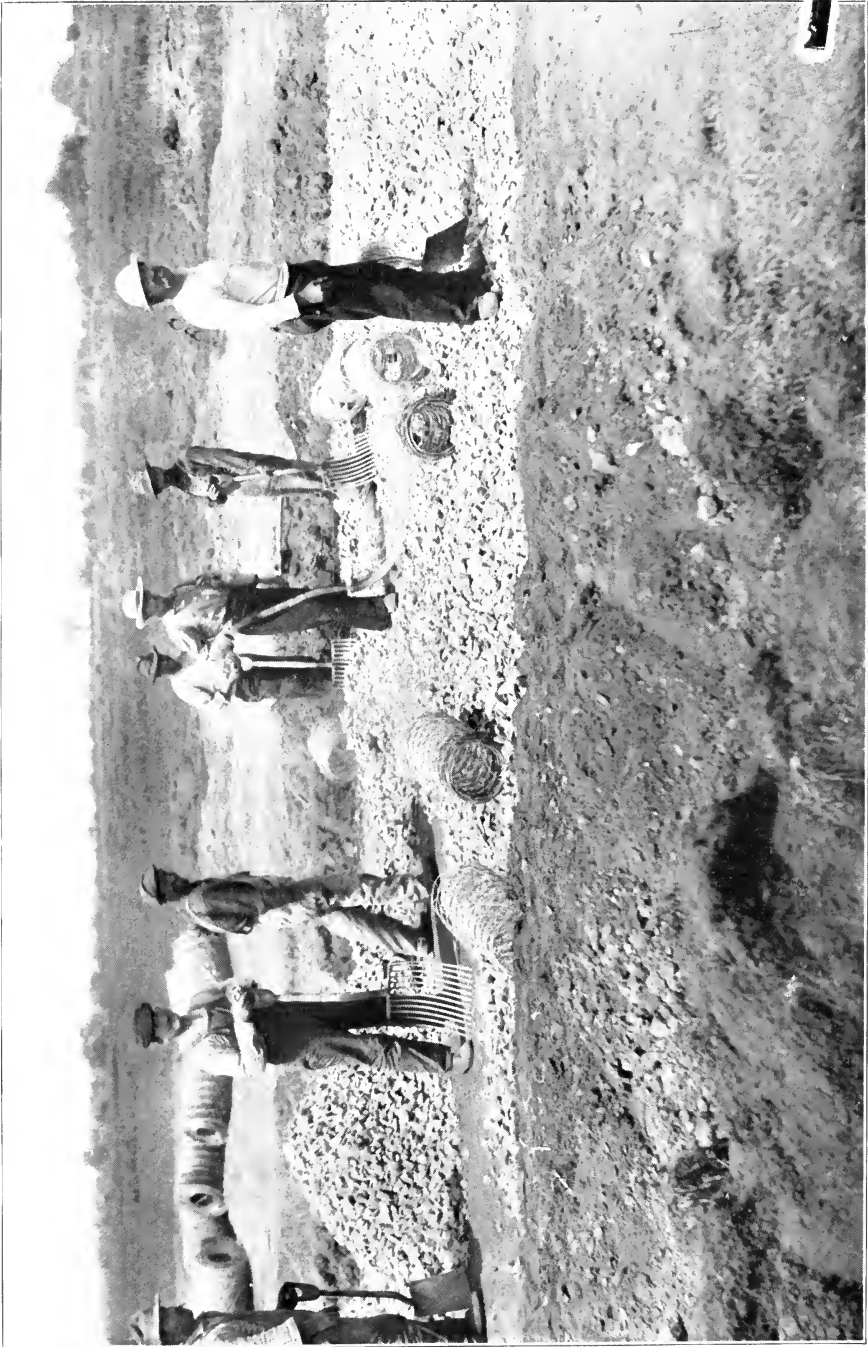
Long Island Motor Parkway. Reinforced Hasam Pavement. Shows Stretching of Triangular Mesh Reinforcement over first layer of broken stone and being covered by second layer of stone.
