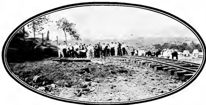
Site of the Gatun Dam—A view across the valley on the line of the proposed embankment 7,700 feet long and one-half mile thick at the base.
