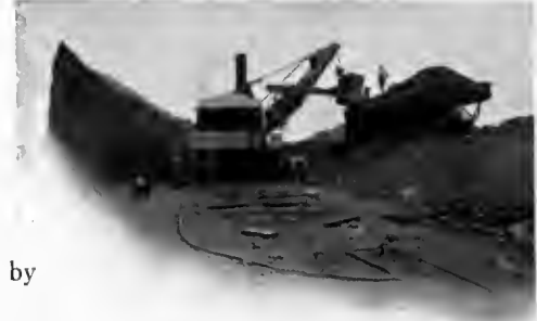
On Gatun Hill—A Steam shovel working in clay on the site of the locks.
