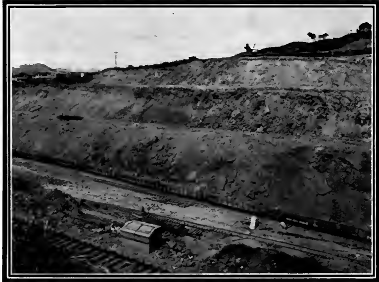
Culebra Cut—The benches or levels by which the excavation is widened. A steam shovel's furrow is forty feet wide.
