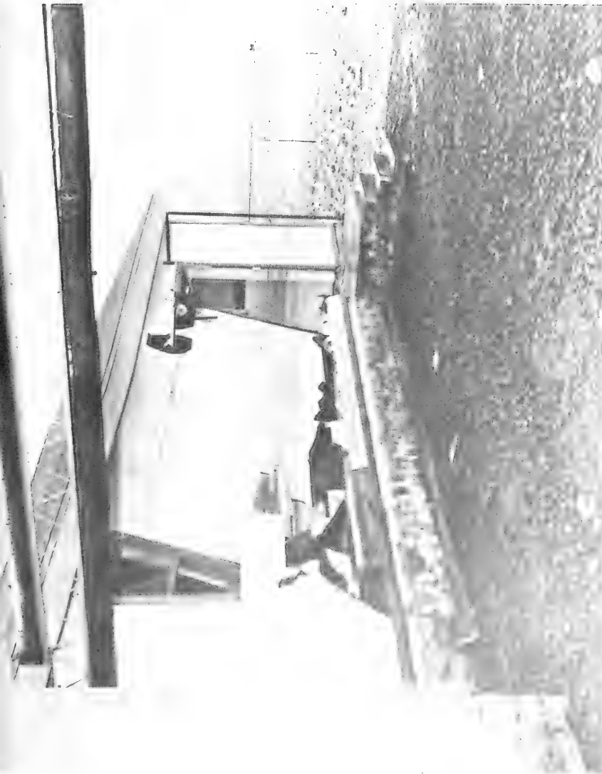
Figure 119 The Ground Electronics Building at Kodiak Naval Station; apparently imploded under Hydrostatic Water Pressure (Photograph by U. S. Navy)
