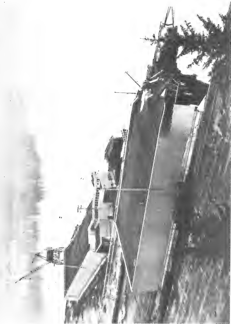
Figure 136 Remains of the Alaska Railroad Docks at the South End of Seward after the Earthquake and Seismic Sea Waves of March 27, 1964. (Photograph by Irvin Cook, Anchorage)
