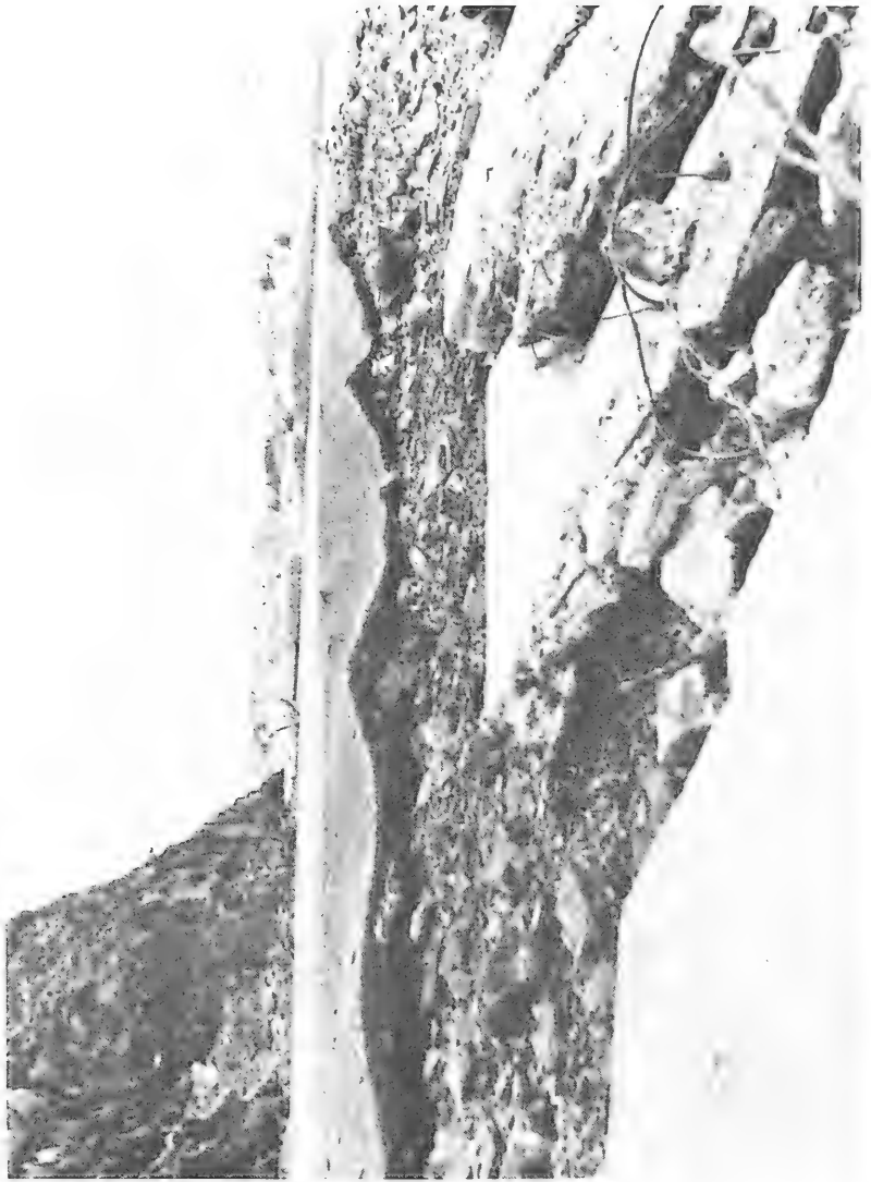
Figure 122 Roadbed Eroded at the Tip of Nyman Peninsula (Photograph by U. S. Navy)
