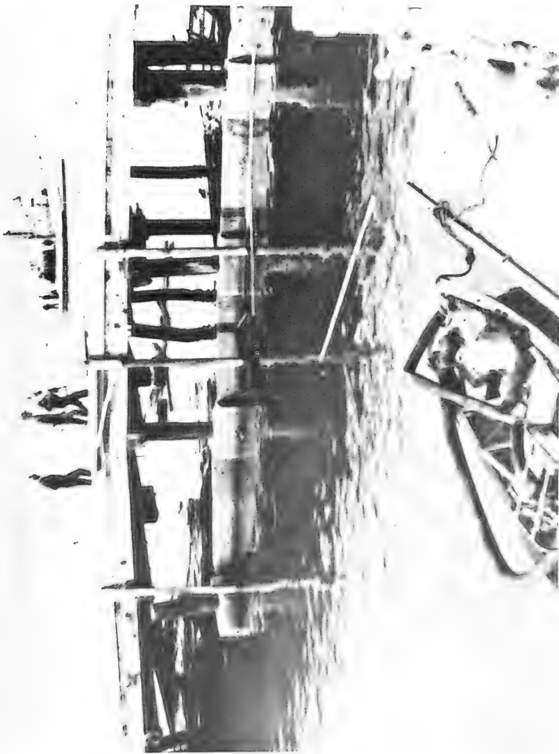
Figure 220 Approach to the Citizens Dock damaged by the Tsunami. Part of the concrete wave barrier surrounding supporting piles has been displaced and torn away. (Photograph by Orville Magoon, San Francisco)
