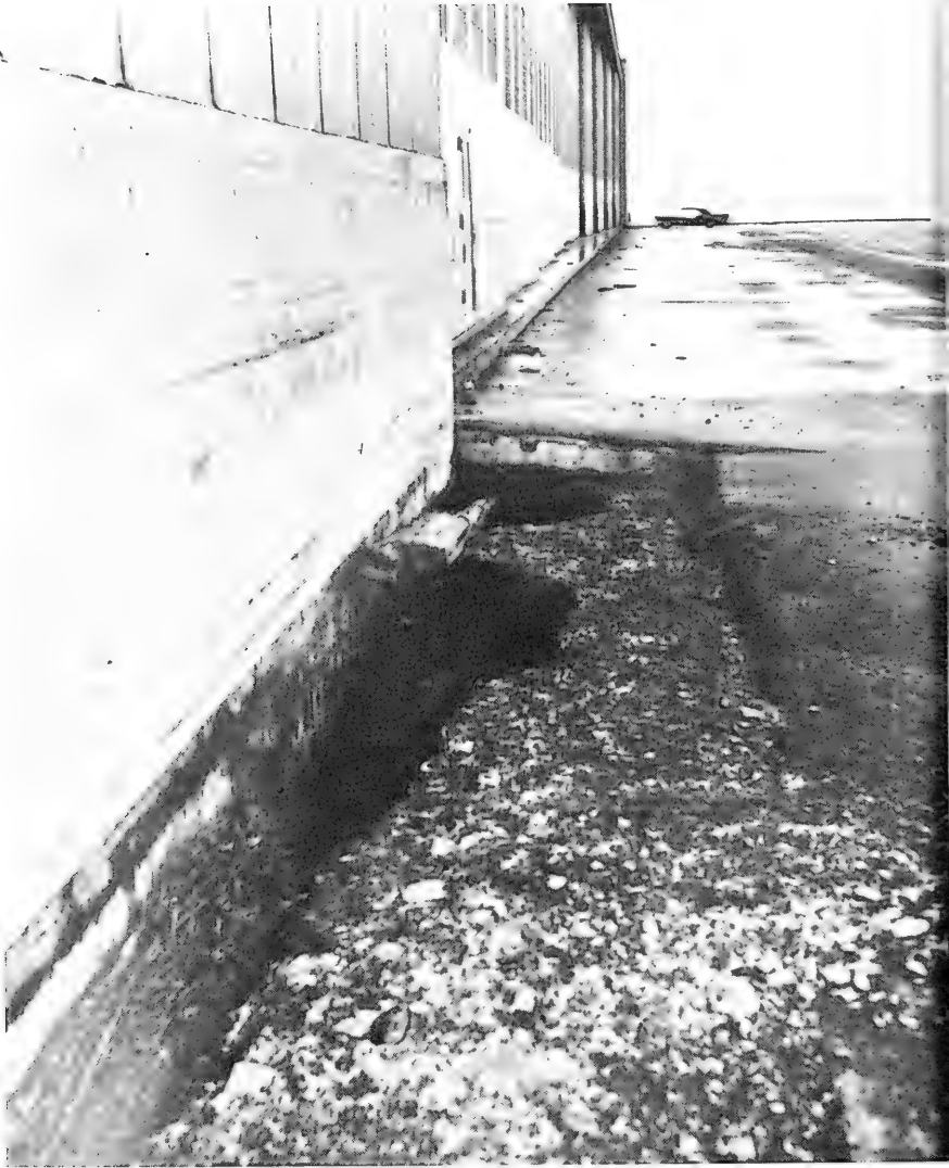
Figure 121 Evidence of Settlement of Backfill Material below Pavement Level, adjacent to the foundation of a Hangar at Kodiak Naval Station. (Photograph by U. S. Navy)
