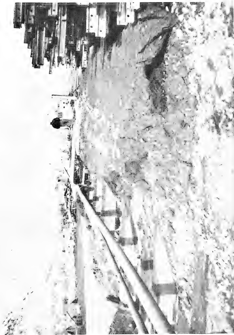
Figure 183 The eroded approach ramp to the North Dock. (Photograph by U. S. Army)
