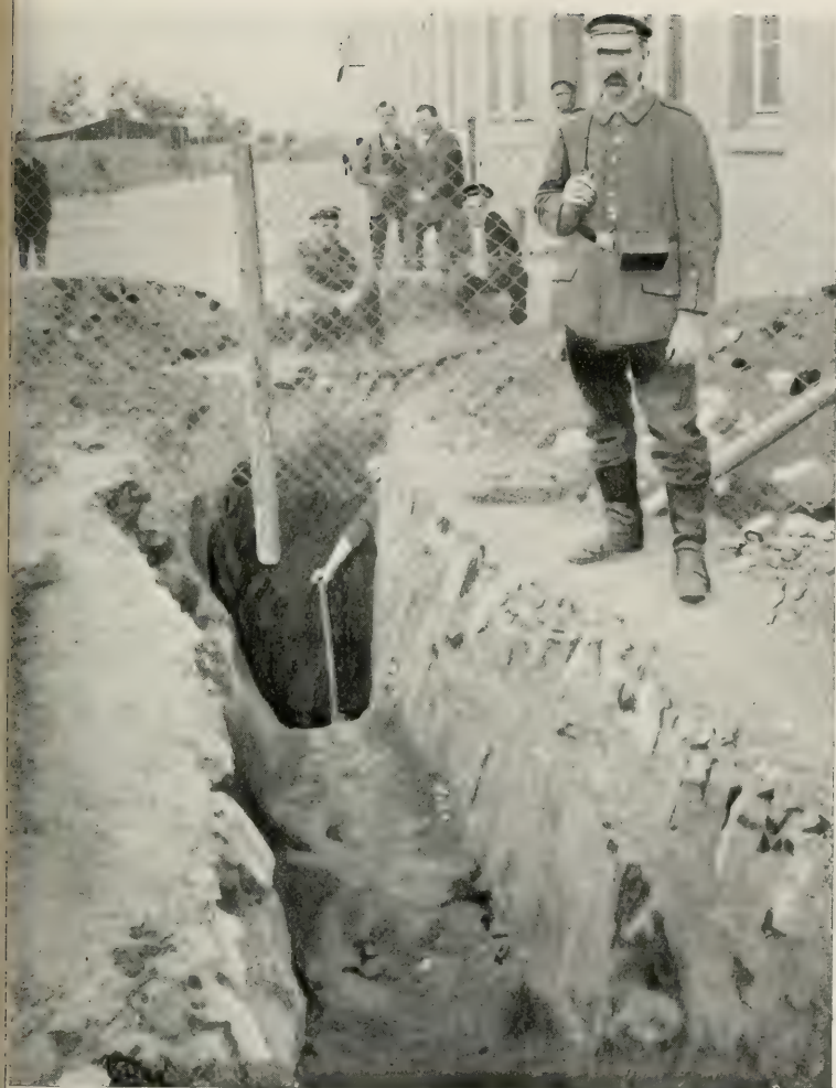
Orderlies digging out the tunnel between Kaserne B and the outer wall.
