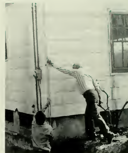
Clare Rose (right) works with architect and construction crews as foundation for the playhouse is dug. Mr. Rose has also been instrumental in getting donated services and goods from local firms.
