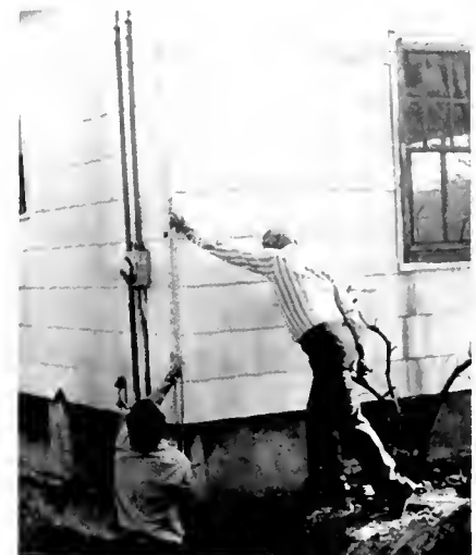
Clare Rose (right) works with architect and construction crews as foundation for the playhouse is dug. Mr. Rose has also been instrumental in getting donated services and goods from local firms.
