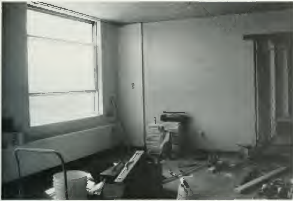
(d) A "before" shot of one of the apartments being under construction this summer.
