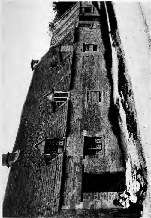
The roof is off the end cottage, the next is boarded up and uninhabited, whilst the nearest one is already doomed. The entire village of Great Rissington is tumbling down in this manner.
