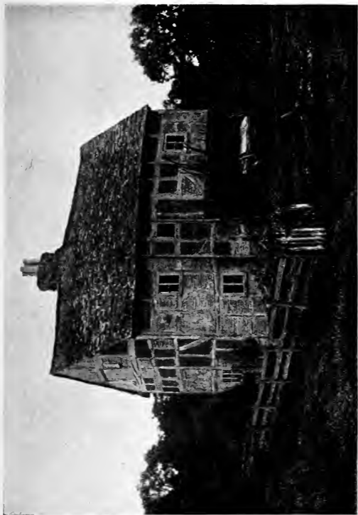
A pair of inhabited cottages on the Duke of Norfolk's estate. Rain comes through the tiled roof and beats through the walls. The windows can only be opened at the risk of the panes dropping out.
