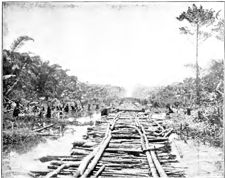
BUILDING RAILROAD THROUGH SWAMP, CORDUROY WITH TIES AND RAILS LAID IN THE BACKGROUND
