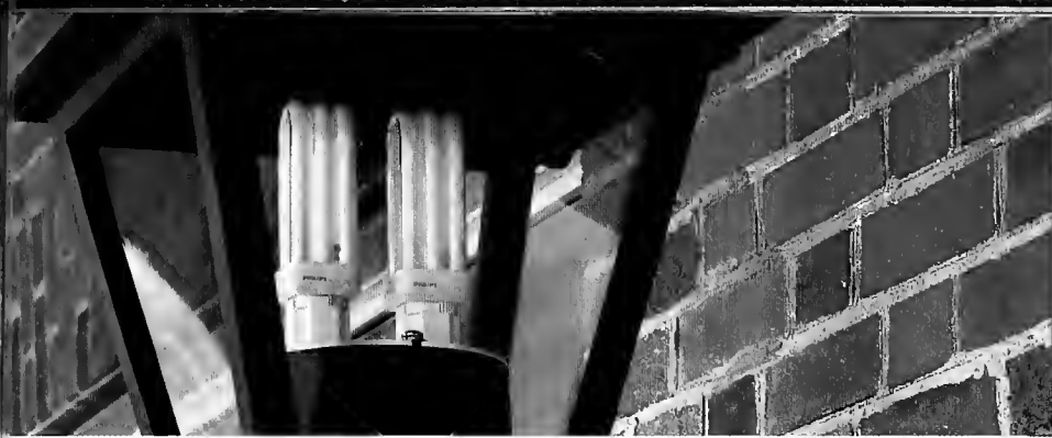
Exterior light fixtures with energy efficient fluorescent bulbs were added as part of the Burney Center renovations.
