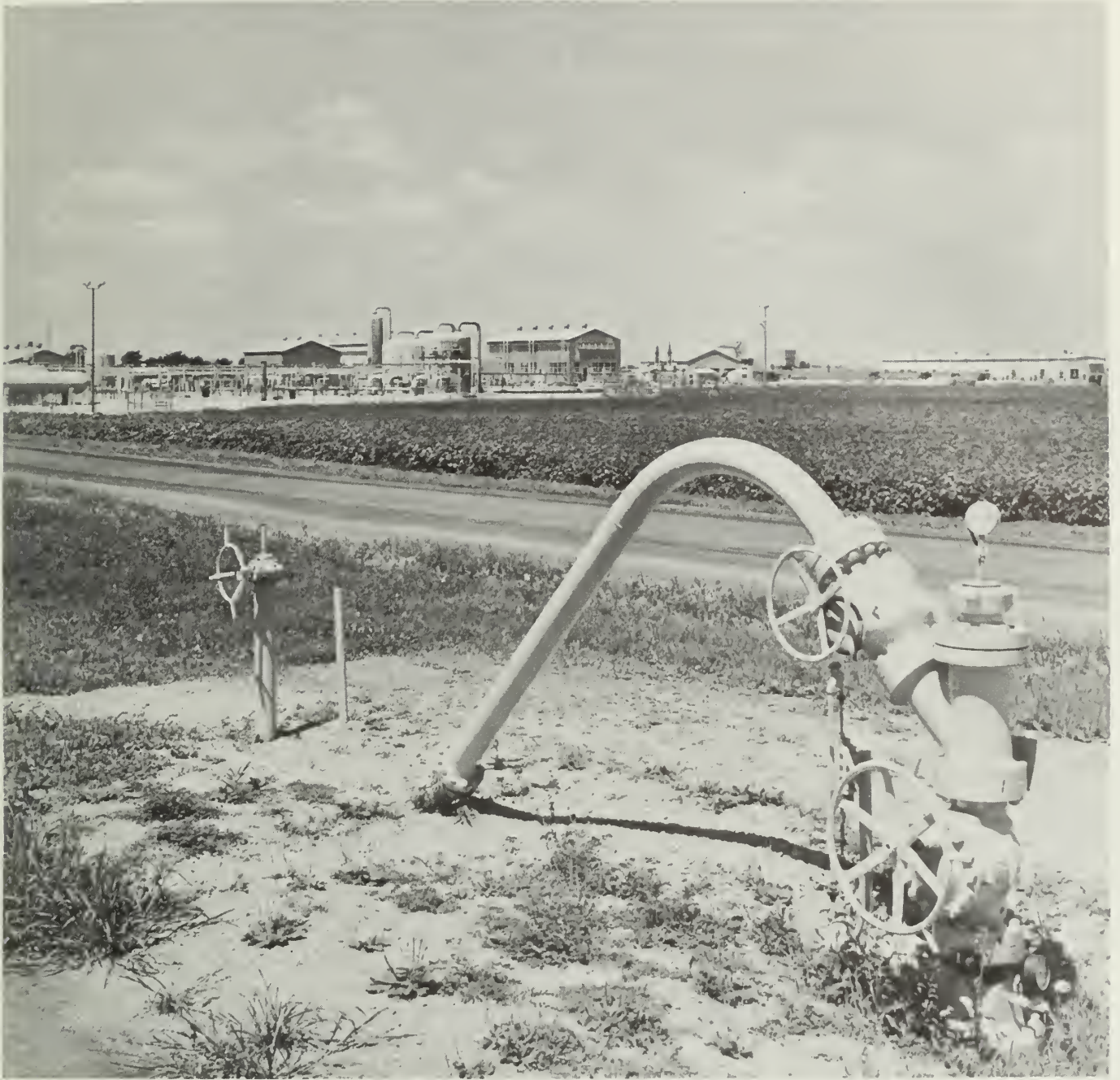
Surface installation for underground gas storage project at Troy Grove, Illinois. Operating well is in foreground; plant for treating and handling gas is in background. (Photograph courtesy of Northern Illinois Gas Co.)
