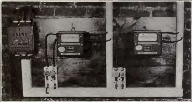
Fig. 132.—Service box with meter loop in wood moulding.
