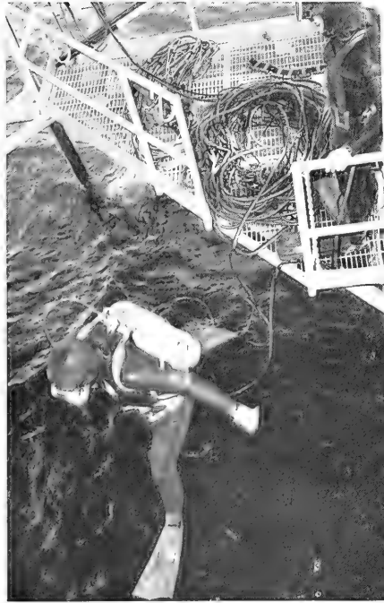
Diver descends from the diving platform to install sea-floor instrumentation. He is trailing hookah hose containing compressed air at 125 psi.
