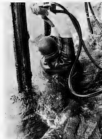
Pneumatic chipping hammers, operated on the same compressed air as the hookah gear, are used to clean marine organisms and other types of fouling from the underwater portions of the tower structure. Excessive fouling adversely affects the normal flow of ocean currents.
