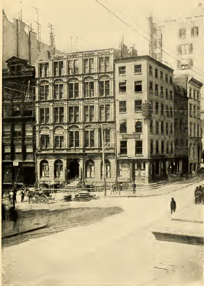
OLD BUILDINGS AT THE CORNER OF WALL AND BROAD STREETS (1885), ABOUT TO BE DEMOLISHED TO MAKE ROOM FOR THE WILKES BUILDING WHICH IN TURN HAS NOW GIVEN PLACE TO THE MAGNIFICENT ADDITION TO THE NEW YORK STOCK EXCHANGE
