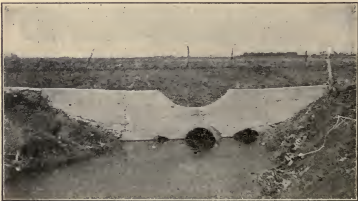
FIG. 7.—A WELL-PROTECTED TILE OUTLET
