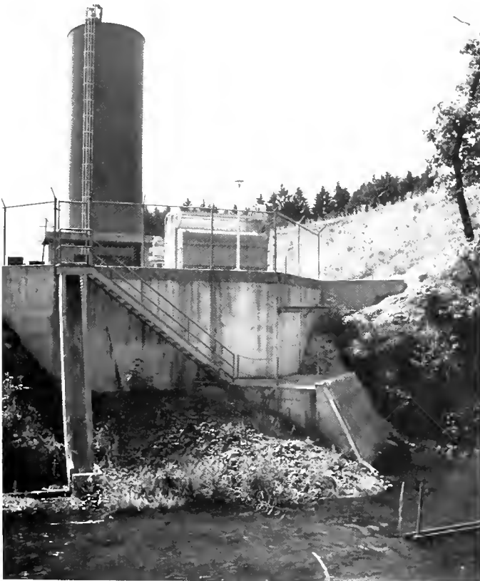
Patton Valley Pumping Plant
