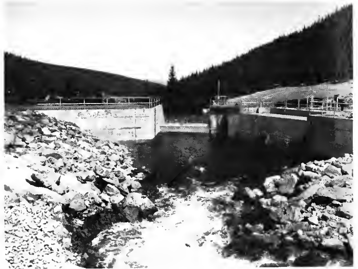
Chapman Diversion, South Side Collection System
