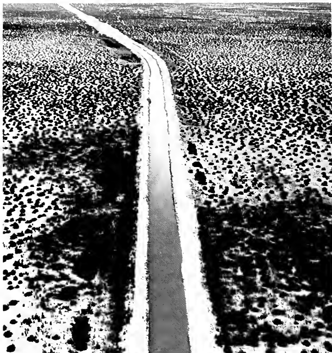
Heavy vegetation growth along unlined section of canal
