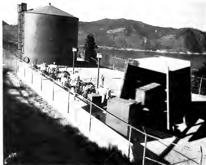
Relift Pumping Plant D, Manson Unit
