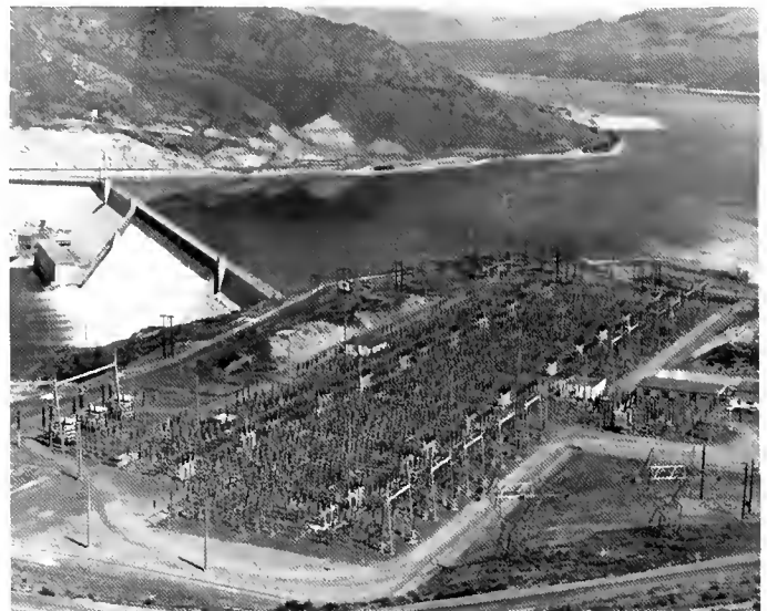
Grand Coulee 230-kV consolidated switchyard
