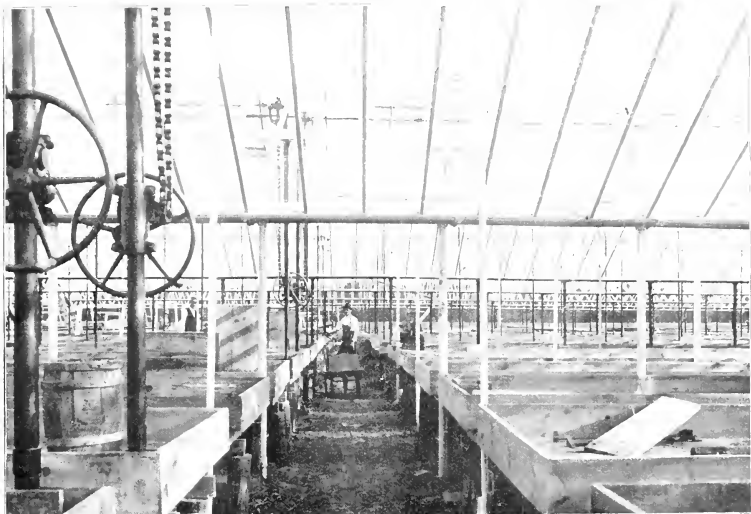
The Garland Iron Gutter and Iron Post Construction in the Houses of A. H. Pochlmann, Morton Grove, Ill. From a Photograph taken last summer during construction.
