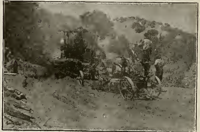
Building the Road up into the Mountains; it now extends for a dozen miles and is a remarkably good mountain road.
