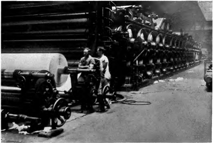
THIS picture shows, from right to left, the long row of dryers, the calendering stack, the winder, and the rewinder of one of The Tribune's paper machines.
