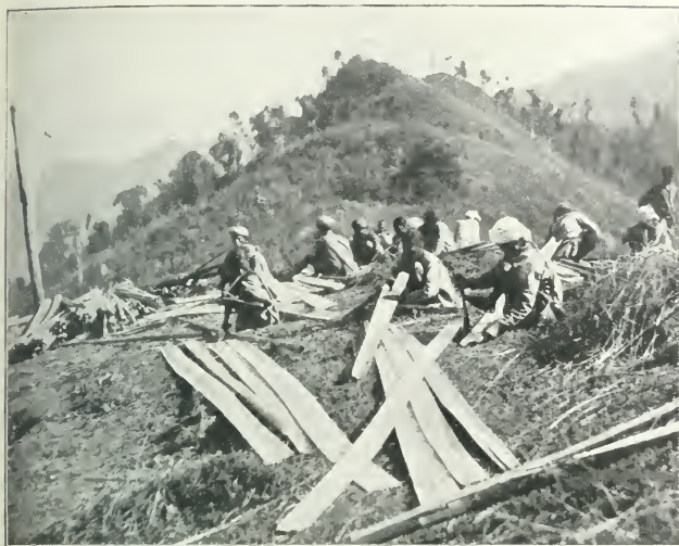
BUILDING A HOUSE FOR THE WHITE VISITORS—"MEN WERE SENT OFF TO GET TREES, BAMBOOS, CANE, AND OTHER NECESSARY MATERIALS." [By the Authors.]
