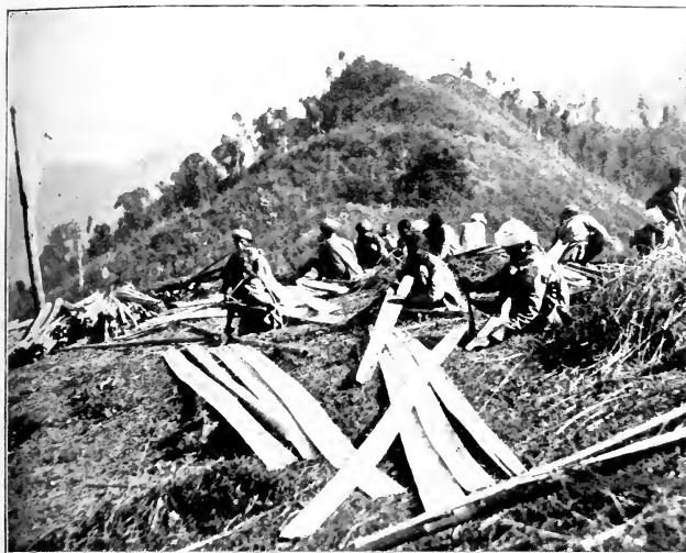
BUILDING A HOUSE FOR THE WHITE VISITORS—MEN WERE SENT OFF TO GET TREES, BAMBOO, CASE, AND OTHER NECESSARY MATERIALS. (By the Authors.)
