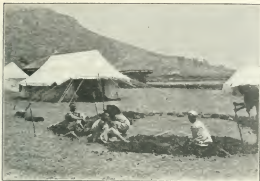
HOW ABYSSINIAN MEN BEGINS TO DIG THE FOUNDATIONS OF A HOUSE. [Photo.]
