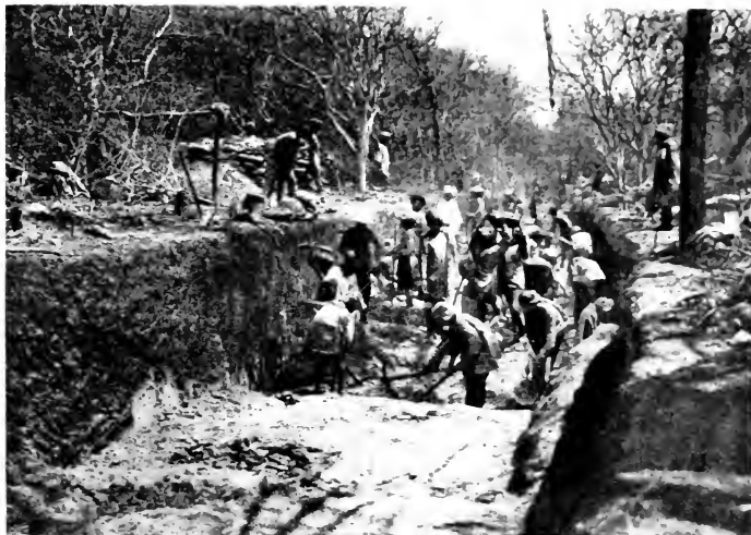
HOW THE WORK IS DONE AFTER A SECTION OF THE RAILWAY HAS BEEN CUT THROUGH.
