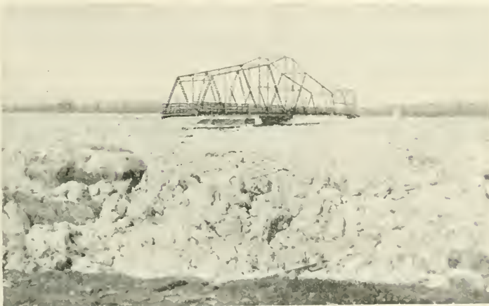
THESE SPANS BELONGED TO THE DAWSON COUNTY BRIDGE, MONTANA. THEY WERE LIFTED OFF THEIR SUPPORTS BY AN ICE-PACK AND CARRIED SEVERAL MILES DOWN STREAM. From a Photo.
