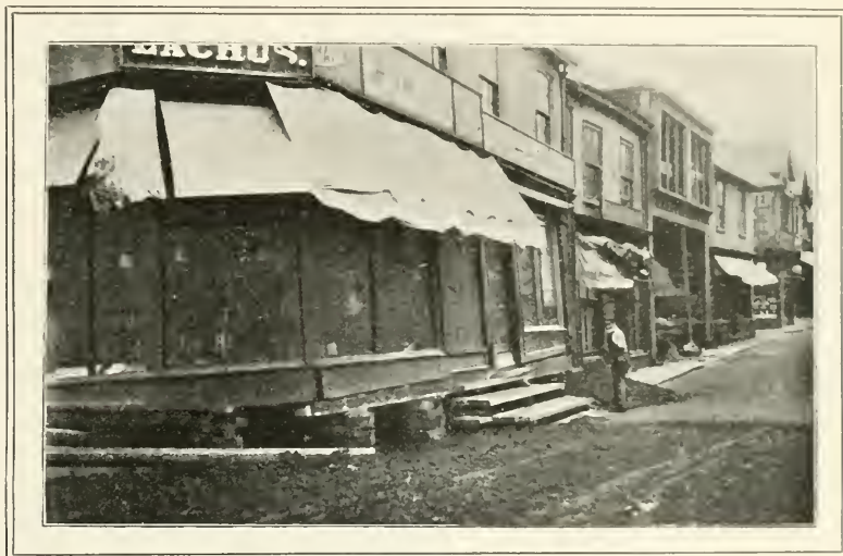
"BUSINESS CARRIED ON AS USUAL"—A SHOP BEING RAISED ON TEMPORARY PROPS WITHOUT ANY CESSATION OF BUSINESS. (Photo. From a)
