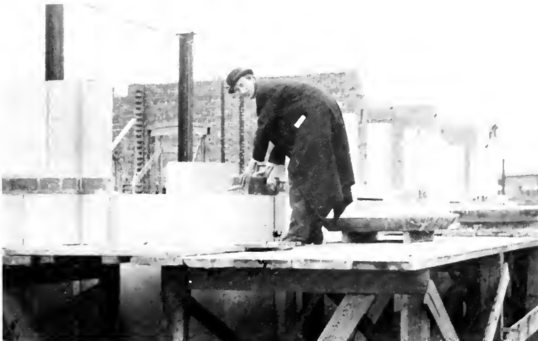
The construction site of one of the original Rice buildings being inspected by the meticulous Mr. Watkin, circa 1911.
