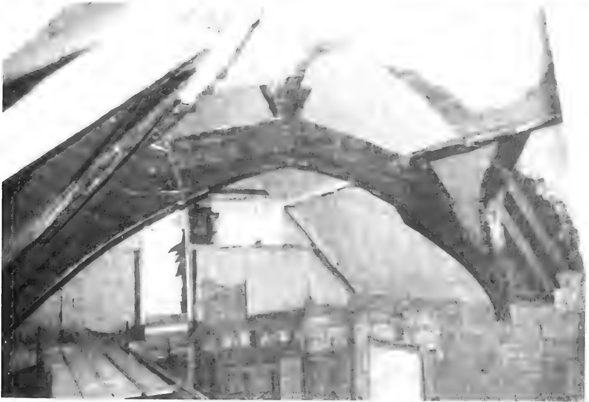
Figure 2. Manor House, Upton Scudamore. The central open truss of the ball from NW.
