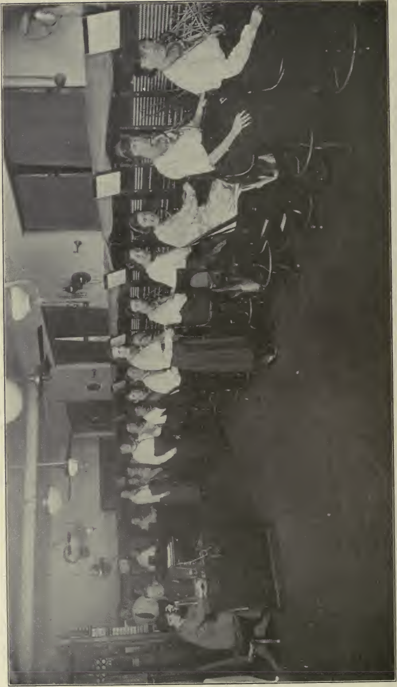
TELEPHONE EXCHANGE, PORT OF EMBARKATION, HOBOKEN, N. J.
