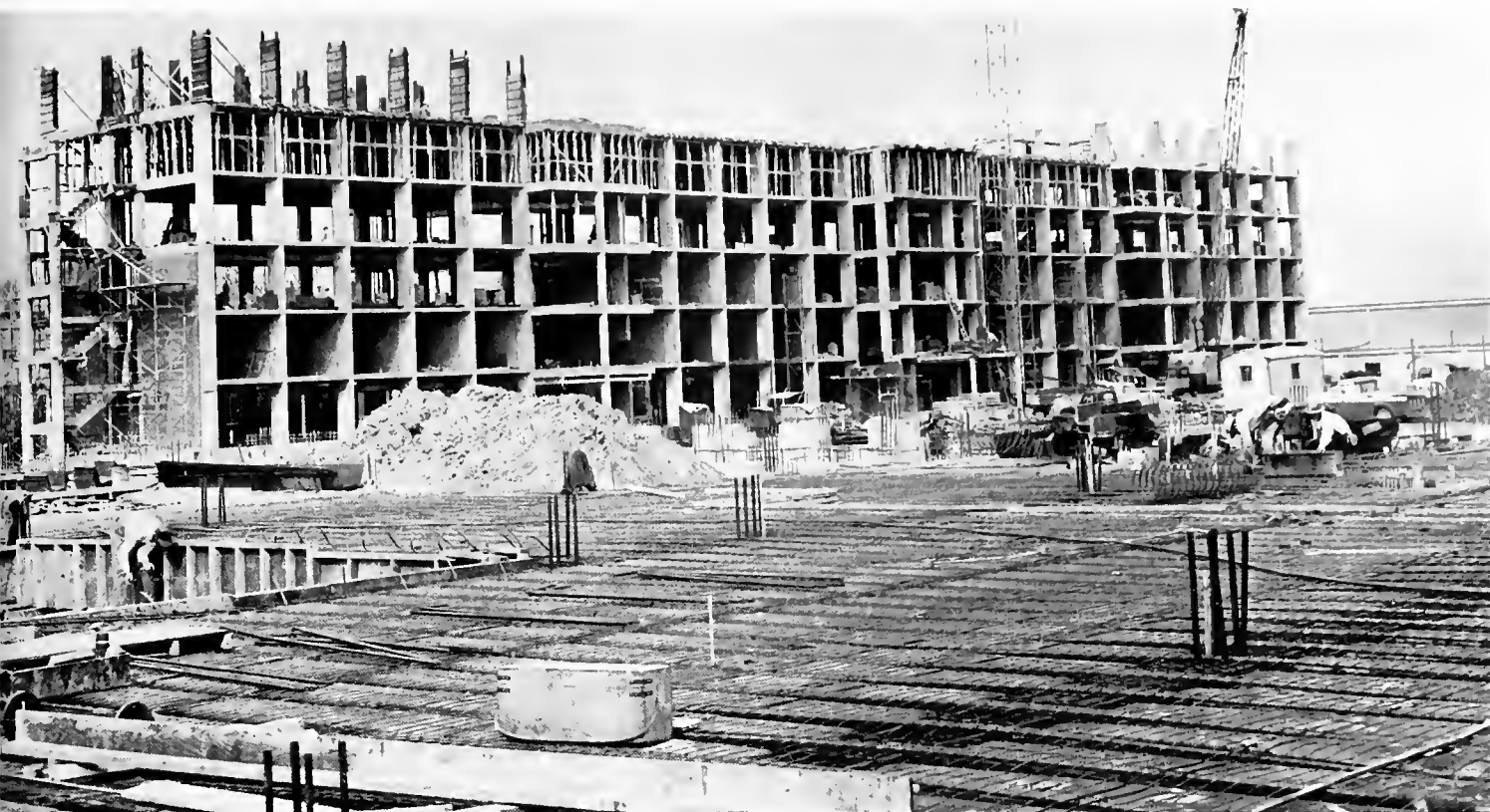
The design of the new campus buildings will be modern and in sharp contrast to that of the existing ones. Here the men's dormitory raises to its sixth floor. In the foreground is the student center under construction also.
