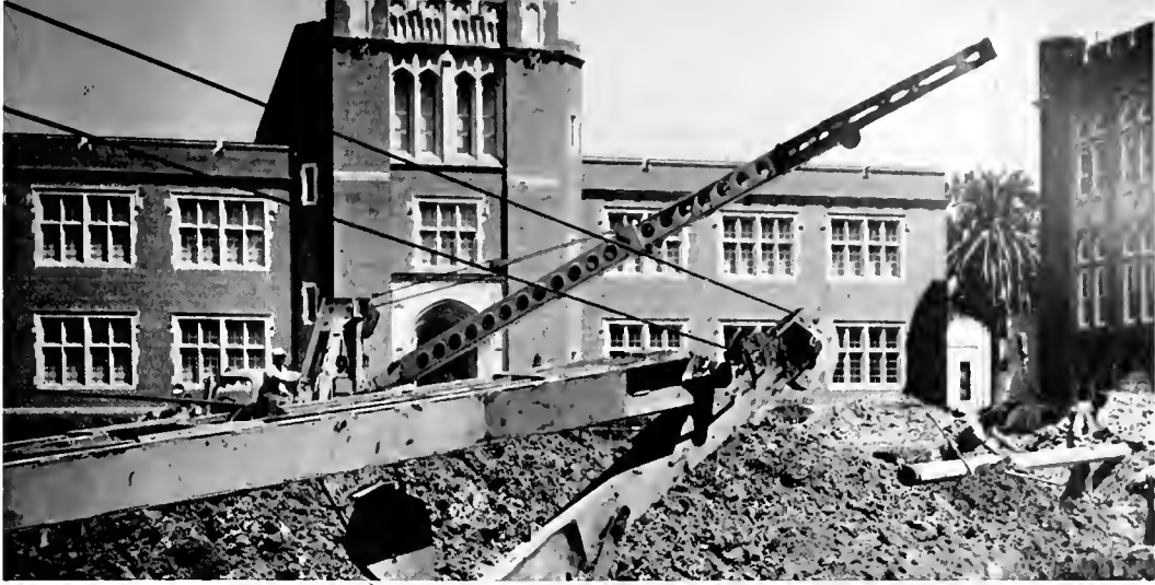
The quadrangle was quite a horrid sight last summer when construction crews laid underground pipes from the new central air conditioning unit.
