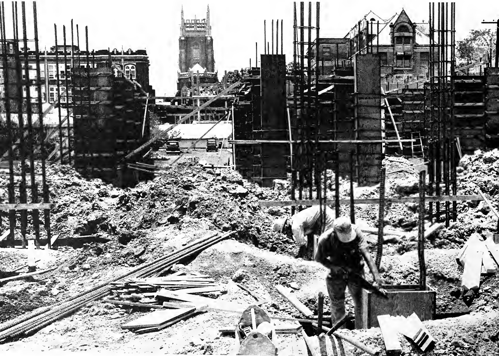
Silhouetted against a background of sky and campus, construction workers drive in the pilings for the foundation. Workers labored under a hot August-September sun to finish the groundwork for the buildings.
