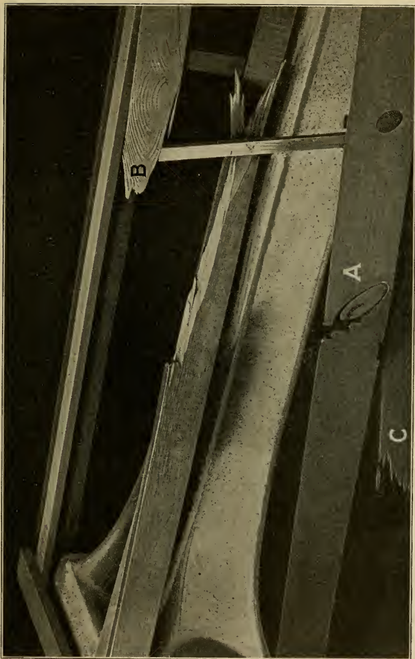
FIG. 15—Broken crating of ornamental concrete lighting post. A. Knot. B. Cross grain. C. Decay.
