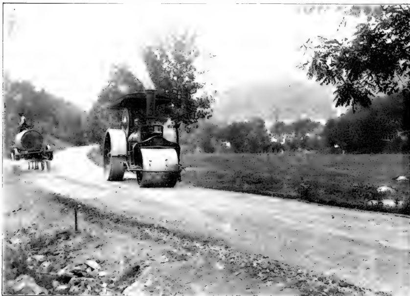
FIG. 2.—FINISHING TOUCHES TO THE SAMPLE ROAD BUILT AT HOT SPRINGS, VA., UNDER THE AUSPICES OF THE OFFICE OF PUBLIC ROAD INQUIRIES OF THE DEPARTMENT OF AGRICULTURE.
