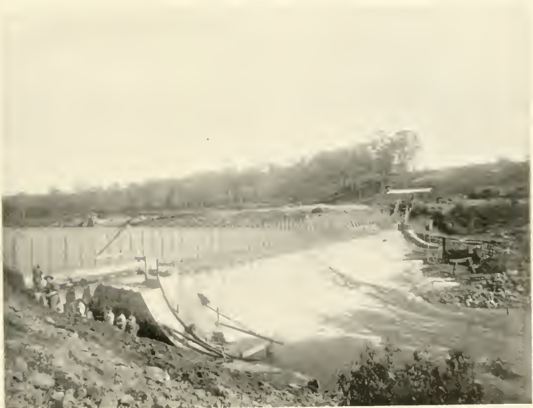
SAMP MORTAR DAM, UNDER CONSTRUCTION, BUILT FOR THE BRIDGEPORT HYDRAULIC CO., AT FAIRFIELD, CONN
