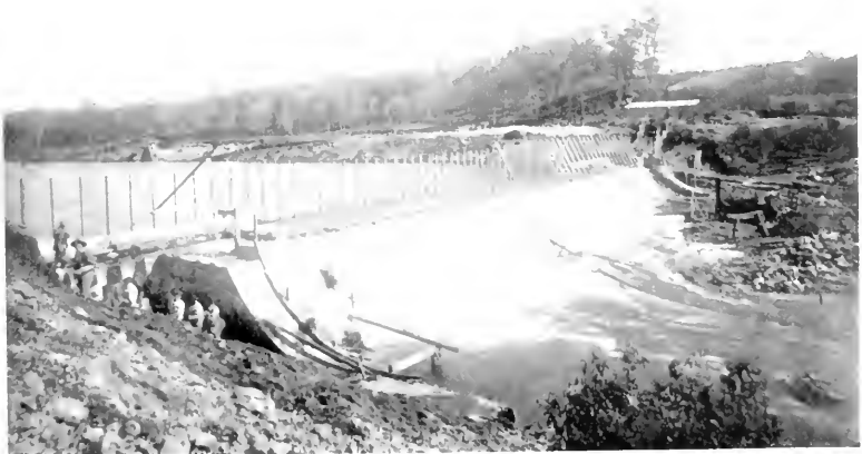
SAND MORTAR DAM, UNDER CONSTRUCTION, BUILT FOR THE BRIDGEPORT HYDRAULIC CO., AT FAIRFIELD, CONN
