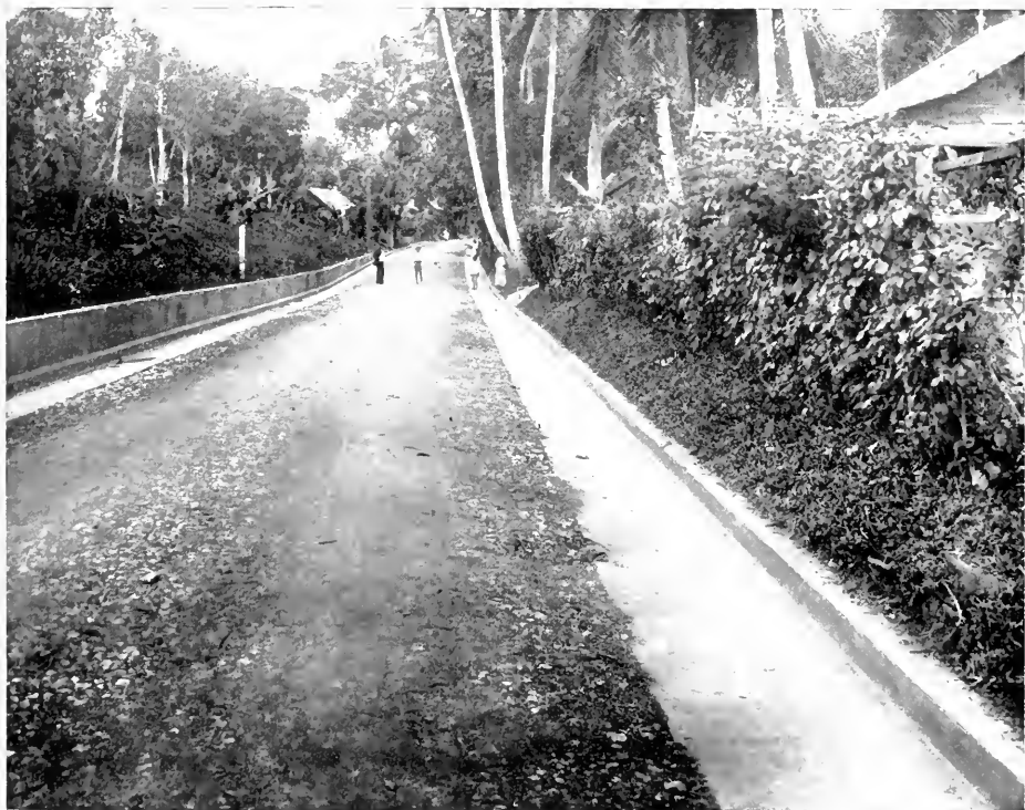
FIG. 57.—A Road in Port of Spain, properly graded, with well-made concrete side drains.
