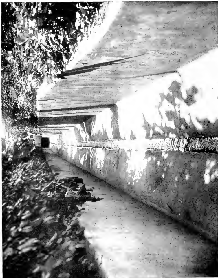
FIG. 3.—The Bed of a Water-course, made in concrete, to prevent the formation of puddles and the breeding of mosquitos. Trinidad, 1909. (From Mosquito or Man? )
