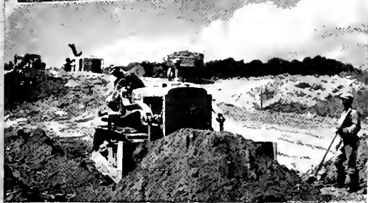
(3) Above — In foreground, International T40 Tractor, and Bucyrus-Erie Bull Grader, at work in Virginia.
