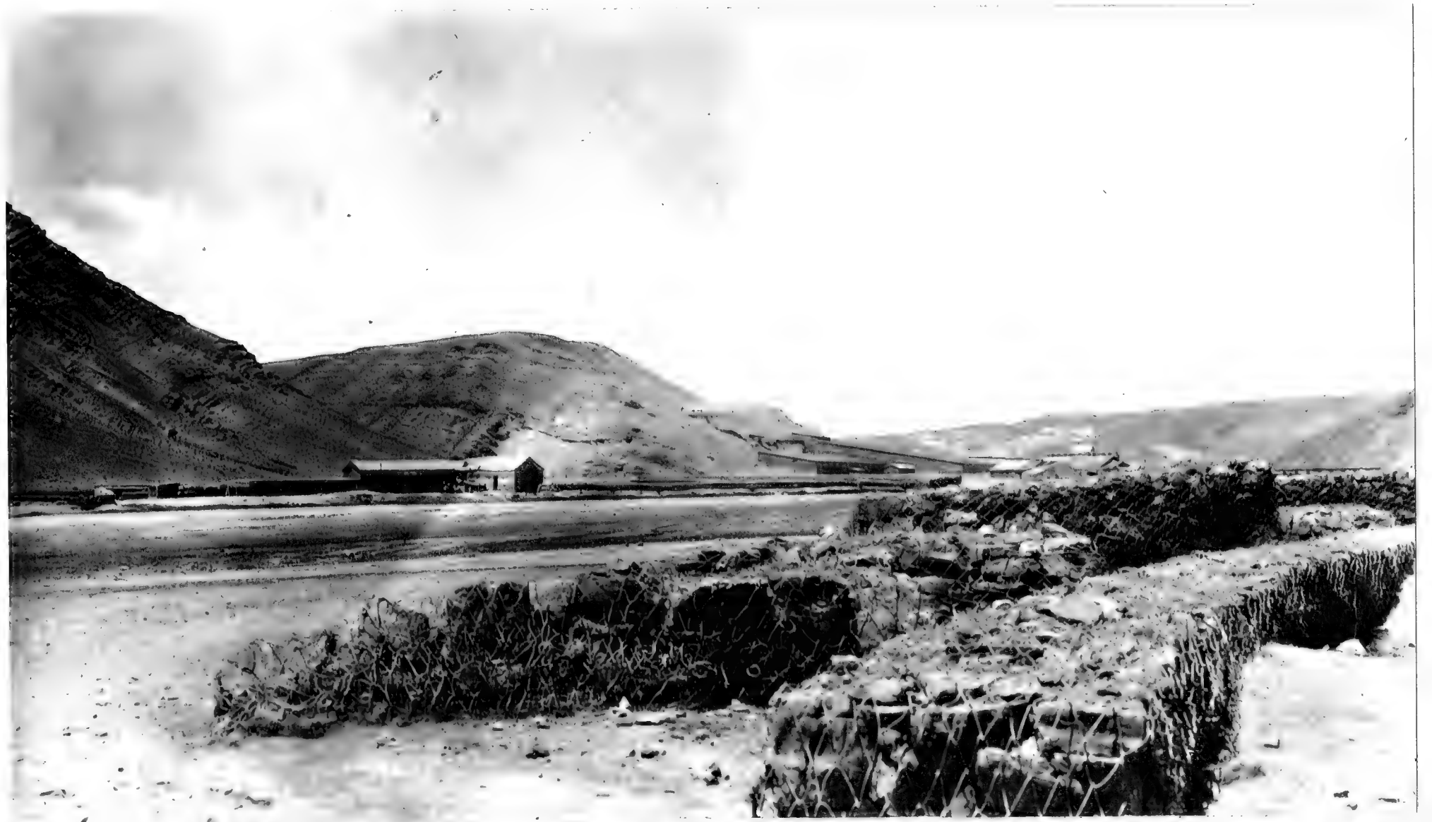
1580. A river bed in the desert region of southern Bolivia, near Atocha. The stones inclosed in heavy wire netting are used to protect river banks against erosion in times of flood.
