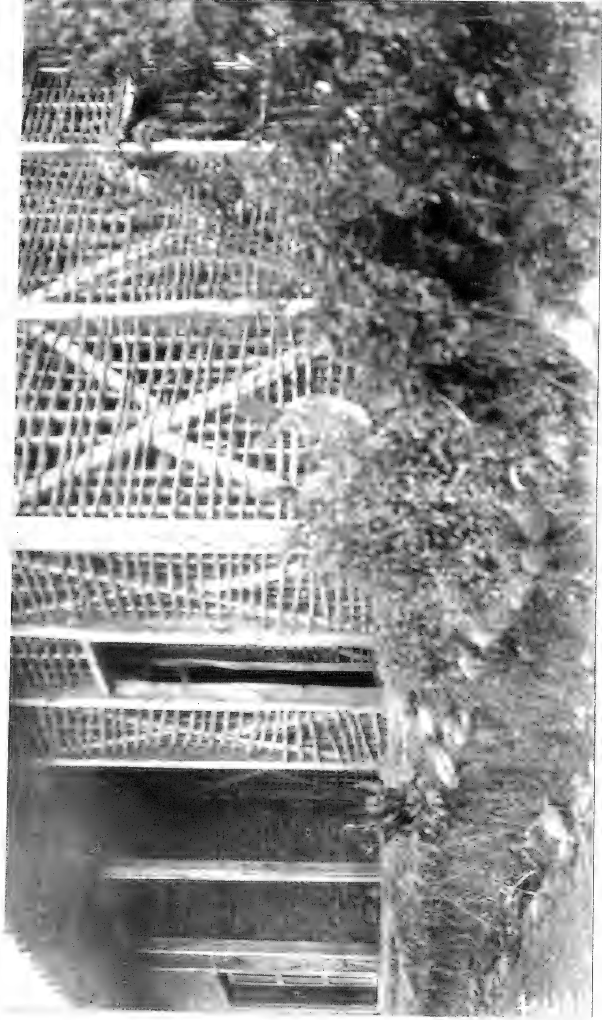
1144. A partly constructed house near Cuenca, Ecuador, showing the frame work. The heavy pieces are of wood, the smaller cross pieces of carrizo ( arundo donax ). a large grass.
