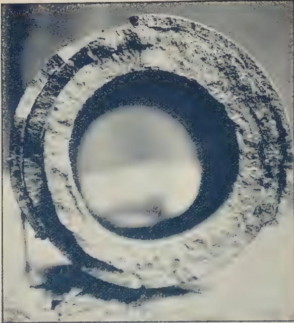
Section from inside of Overflow Pipe to Cistern at 749 feet level in South Star Mine. Principally dolomite carried in solution, with little other matter carried in mechanical suspension. Diameter, about 3 inches.
