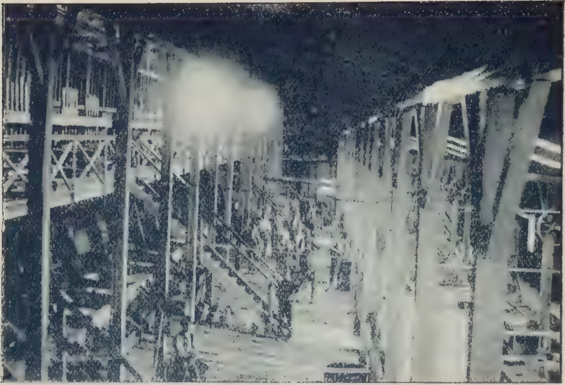
Star of the East Company's Crushing Battery. Inside the eighty head building. (Looking north from the engine-stand).
