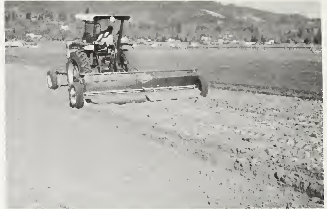
Figure 5 - After application, the dazomet granules are incorporated into the soil and sealed with a roller or water seal.
