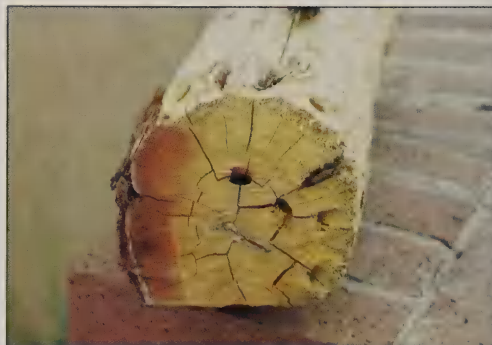
Cross-section of damage.
