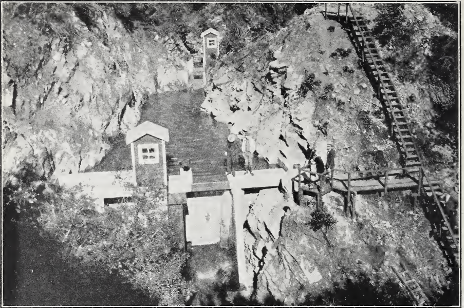
Installation at mouth of Bell Watershed No. 2. Ambursen type dam used to catch eroded material from 101-acre watershed. Gaging station at head of reservoir provides continuous record of run-off. This installation is typical of six controls for Bell and Fern Watersheds.
